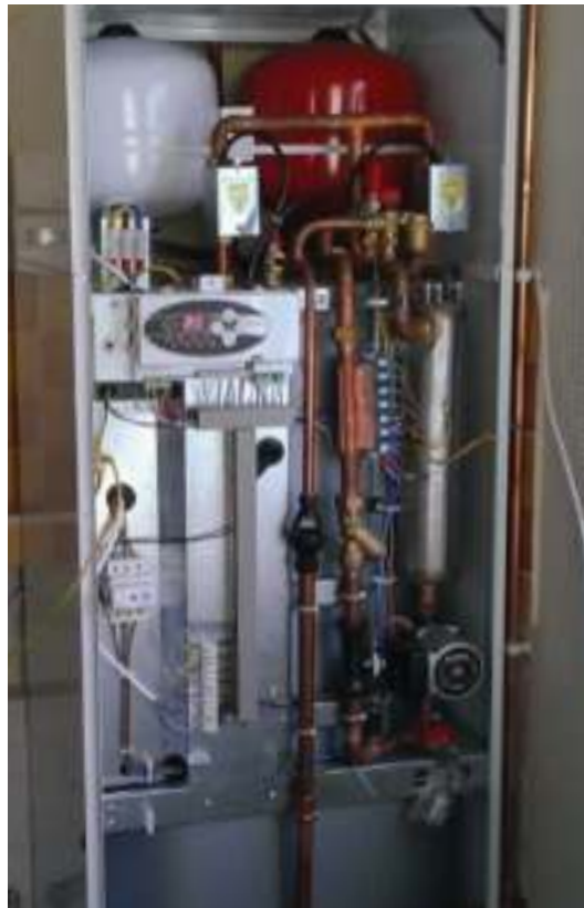
The new EHC Comet was installed in the same location as the previous boiler to minimise disruption
