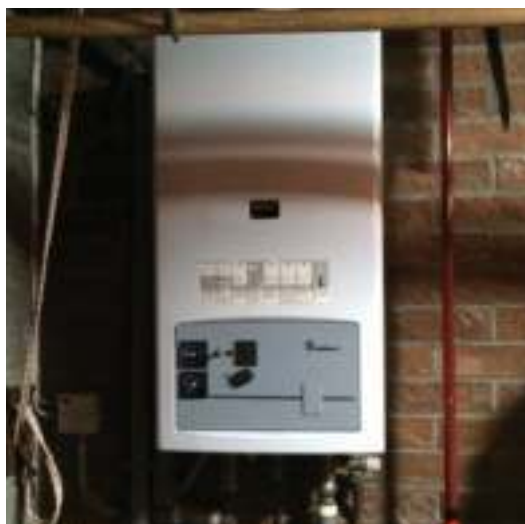
Before and after the installation. The box-off, box-on solution minimises disruption and redecoration.
