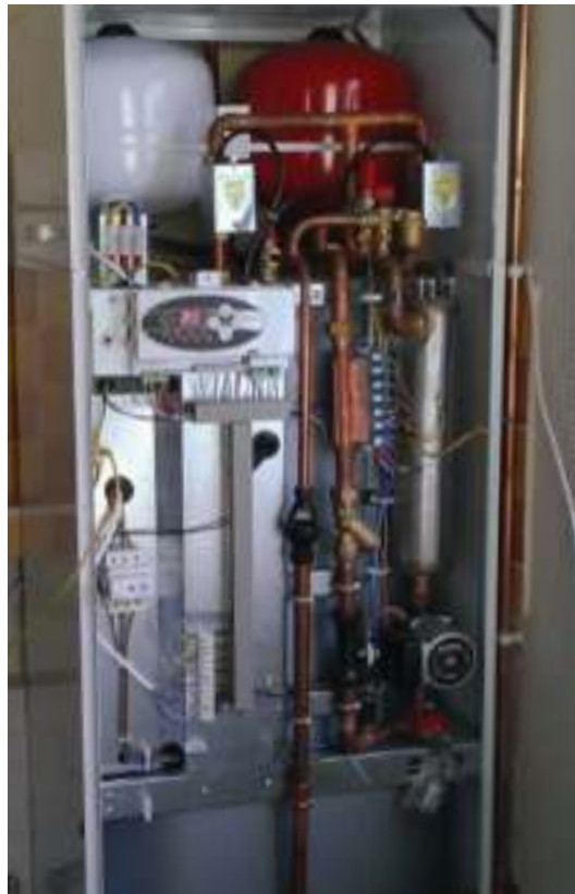
The new EHC Comet was installed in the same location as the previous boiler to minimise disruption
